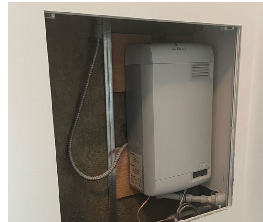
Below: Suite humidifier installed at Tridel at The Well Classic Series I.
